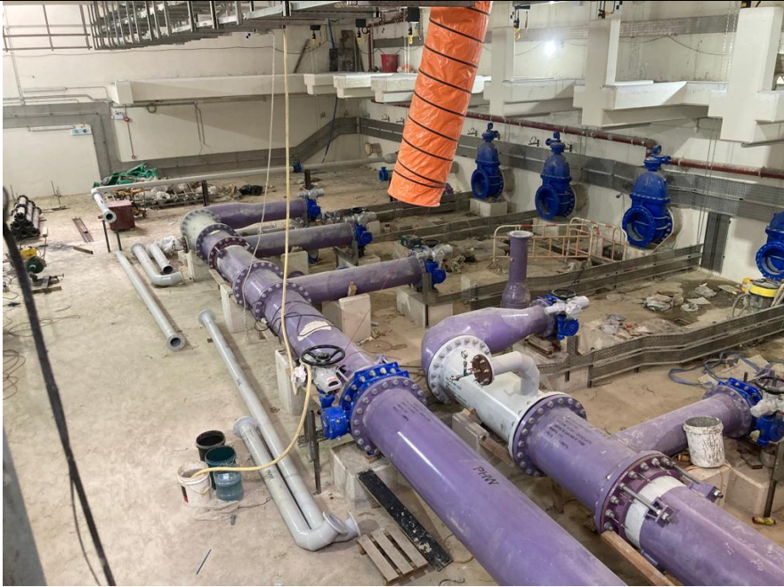
Main pump & associated pipe works at ReWPS Pump Hall
